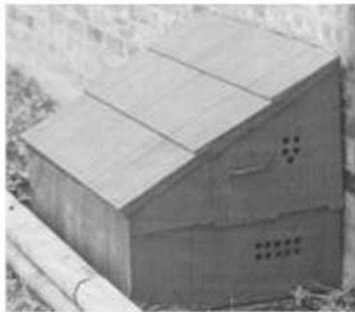
Outdoor housing for the idler motor of the author's rotary phase converter.
